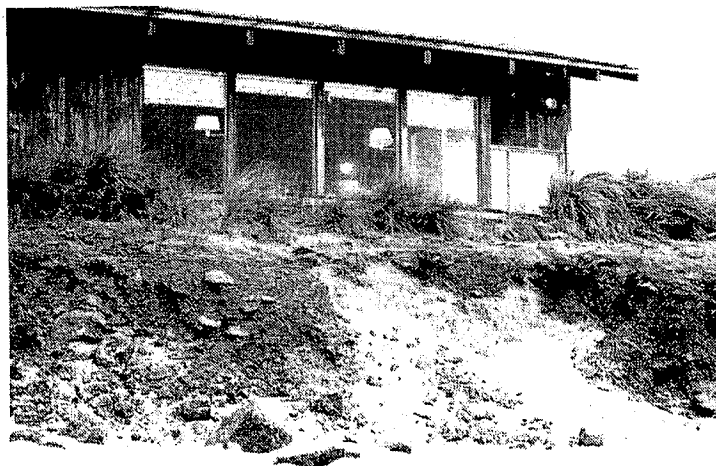
Figure 29. Erosion of riprap on Siletz Spit by a series of storms, exposing the dune sands to wave attack (from Rea and Komar, 1975).
