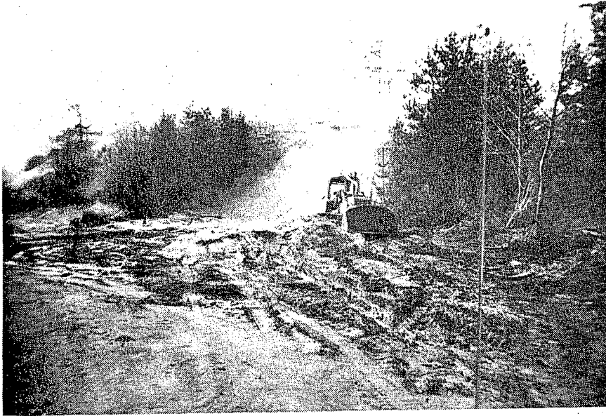
Figure 3. Sand being removed just west of Highway 101 between Glenada and Dunes City. Throughout this stretch of Highway 101, migrating dunes are within several hundred feet of the pavement.
