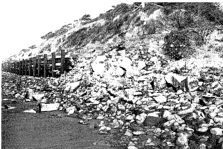
Figure 33. The wood piling bulkhead built on Netarts Spit to stop wave attack of the dunes.
