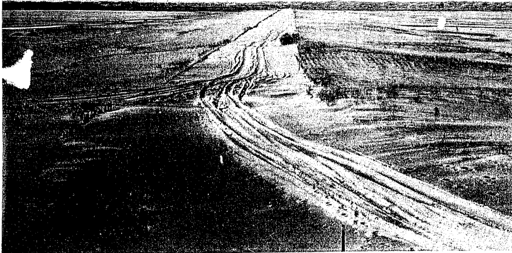
Figure 32. Illustration of sand fencing used to raise a roadbed across a wet deflation plain near Florence, Oregon.
