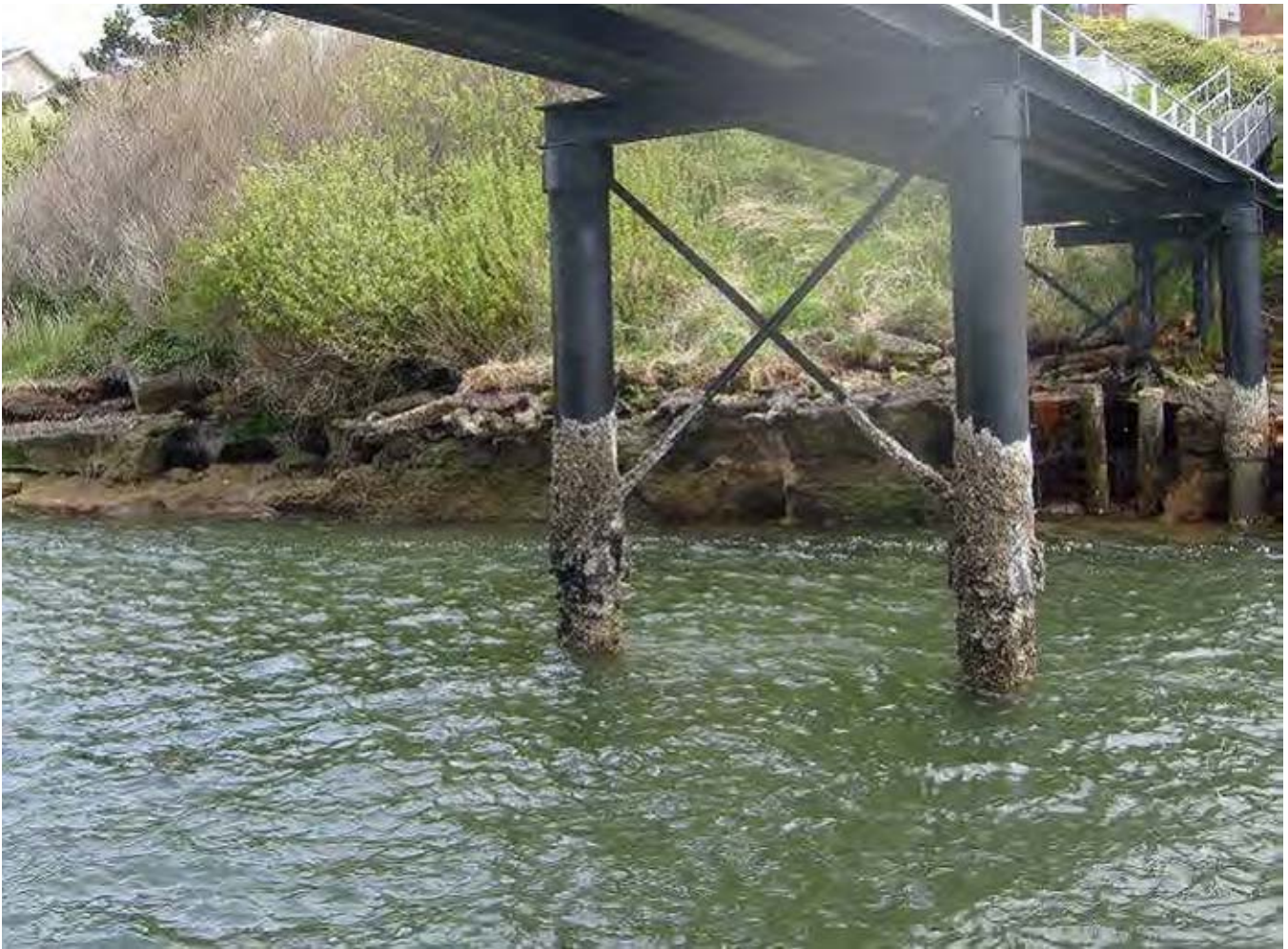
You can see how the piles have become exposed in the one below.
