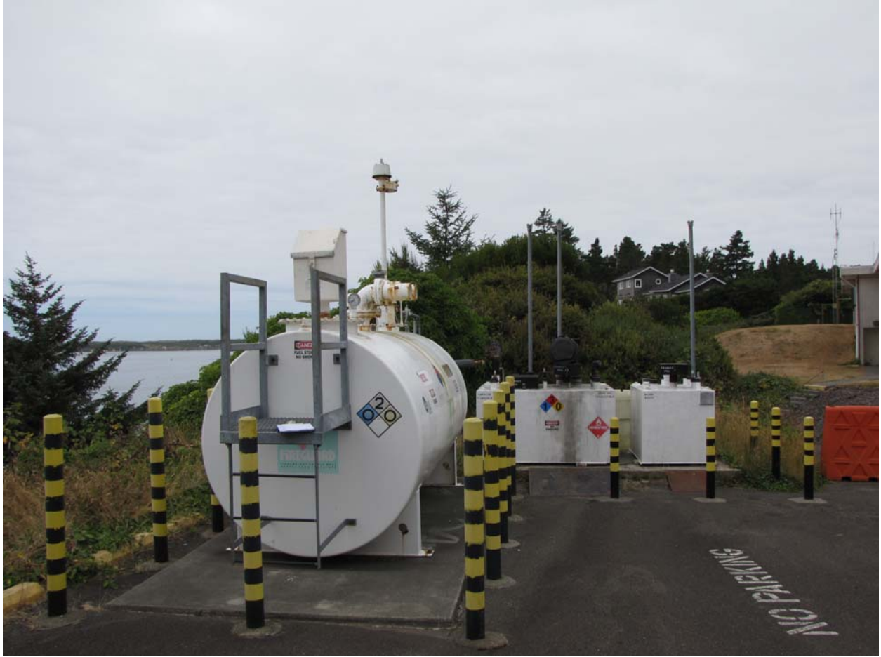
Looking north showing fuel tank storage area.
