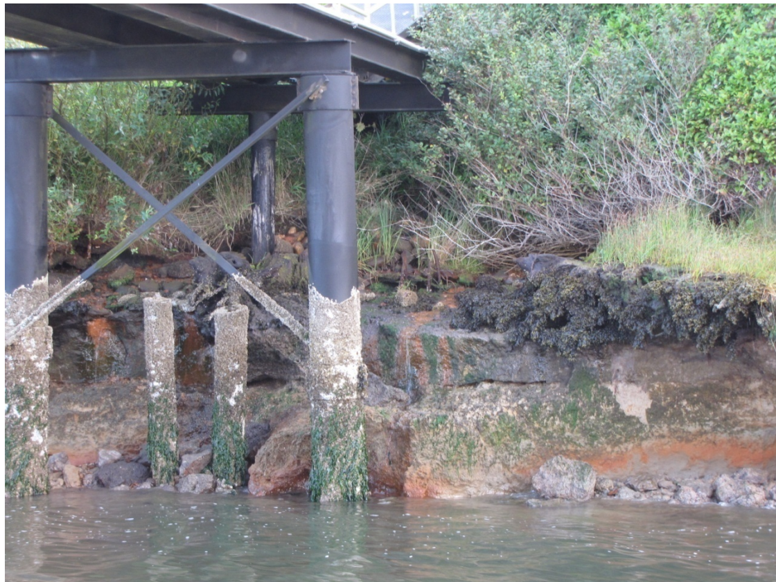
Figure 3. Eroding Shoreline is Visible at Low Tide ( looking east toward shoreline under base of walkway ).
