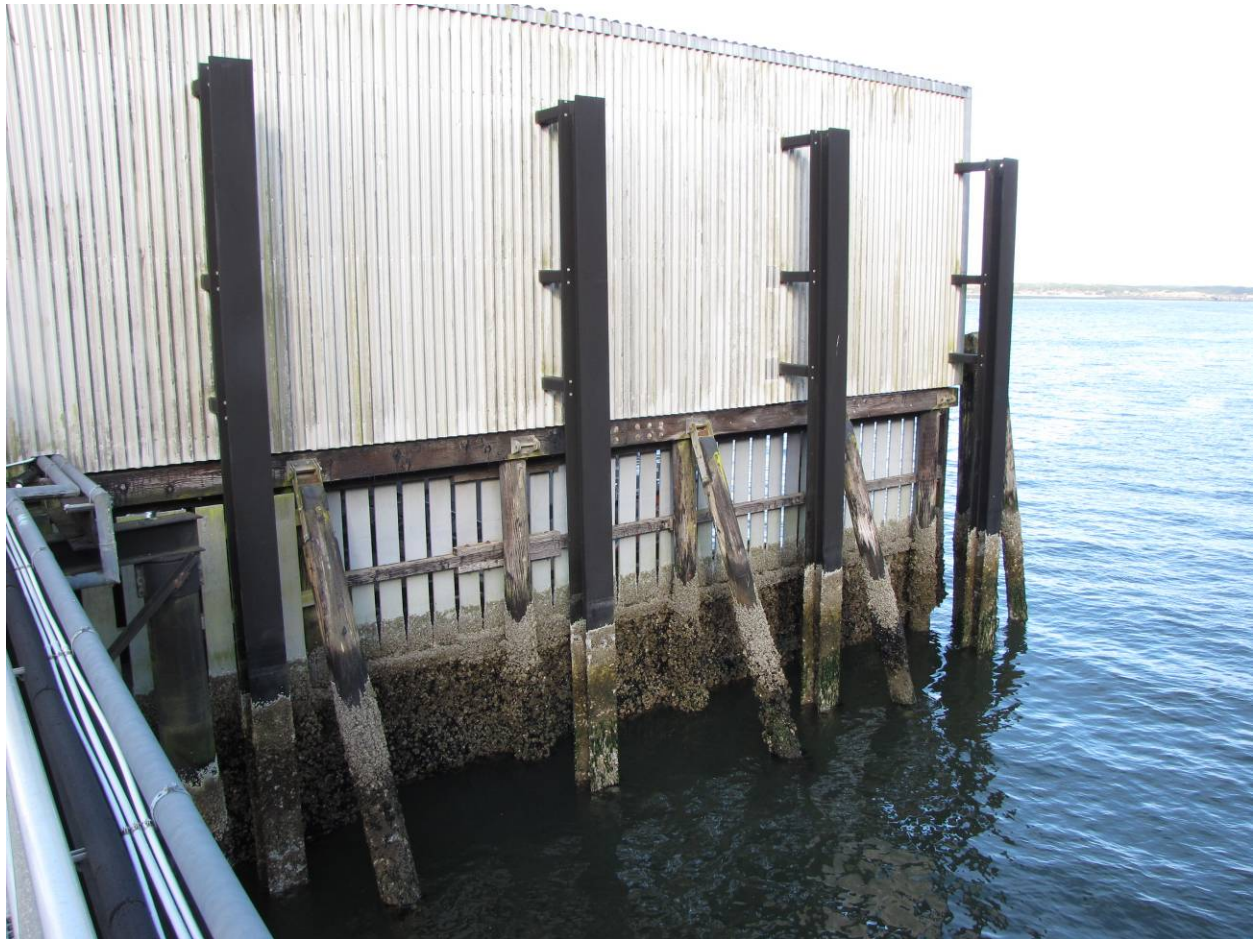
Looking west from walkway along western side of boathouse showing support beams installed in 2008.
