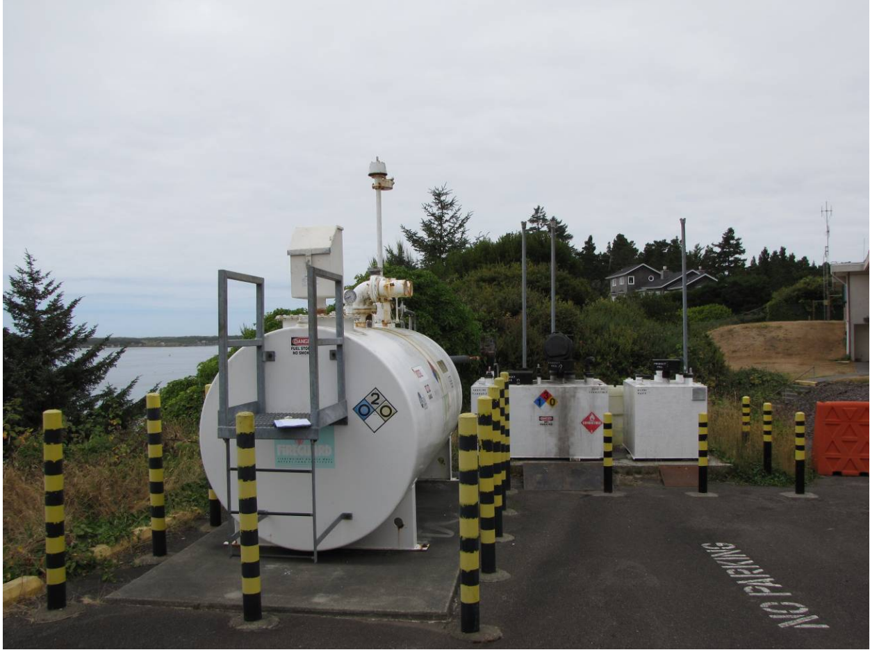
Looking north showing fuel tank storage area.
