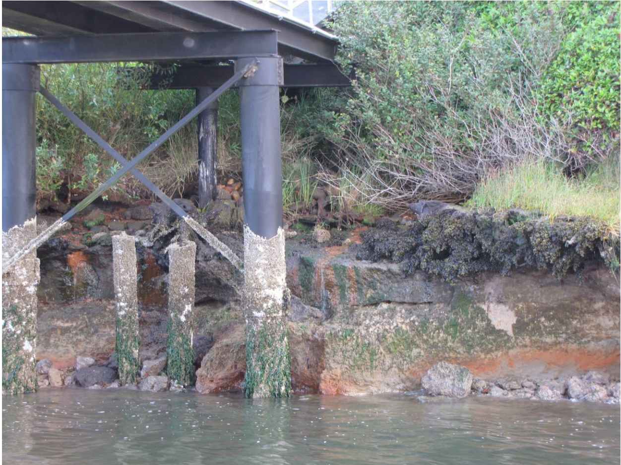
Looking east toward shoreline under base of walkway. Eroding shoreline is visible at low tide.
